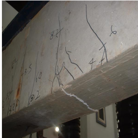
Fig. 14 : Failure mode of beams strengthened with GFRP
