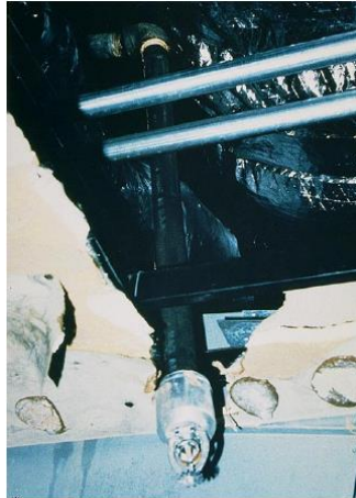
Fig. 1: A sprinkler pipe break at Olive View Hospital [9]
