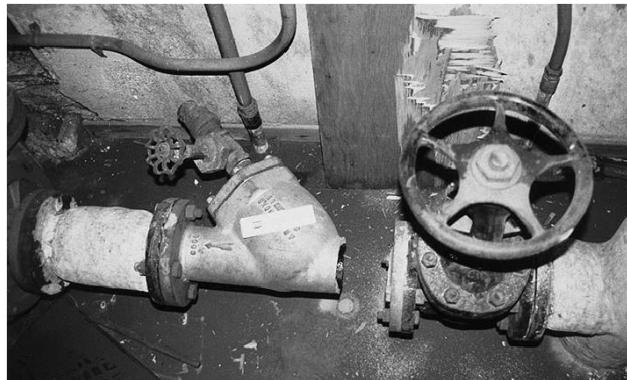
Fig. 2: Four-inch chilled-water lines broke at cast iron valves – Olive View hospital [9]
