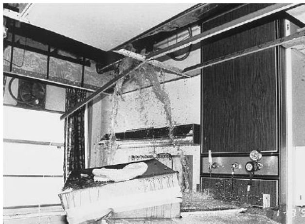
Fig. 3: Extensive flow of water from broken sprinkler pipe at the Sepulveda Veterans Administration medical center, building 3 on the 5th floor [9]
