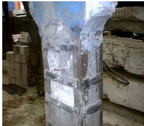
Fig.9: Failure Mode shape for strengthened columns.
