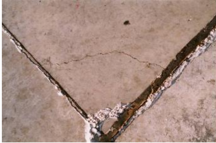
Fig. 2: Circular Cracks Around the Corner of R.C. Slabs & Defects in Expansion and Shrinkage Joints.
