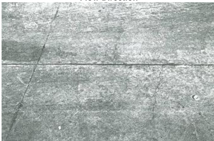
Fig. 4: Cracks Along the Middle of Some Slabs, Parallel to Short Direction of R.C. Slabs and Perpendicular to Traffic Flow Direction.
