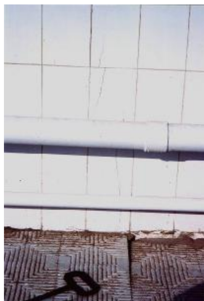
Fig. 6: Cracks in Tiles of End Walls and Separation between End Walls and Floor Tiles, due to Tilting of Retaining Wall Around the Station.
