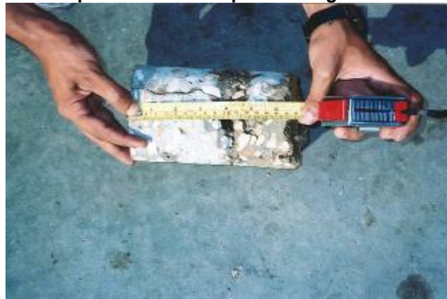
Fig. 11: Sample of Core Test at Cracked Section (Sample # 1), Showing a Total Concrete Depth of 16 cm and RFT Mesh at Depth 10 cm from Top Surface.
