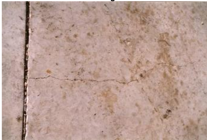
Fig. 3: Cracks Parallel to Short Direction of R.C. Slabs and Perpendicular to Traffic Flow Direction
