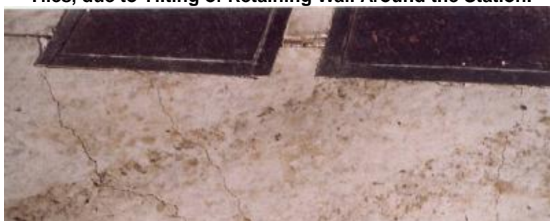
Fig. 7: Cracks Around Electrical and Sanitary Inspection Chambers.
