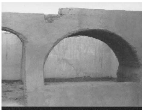
Fig 7: Feliache Project Near Biskra: It Has Been Abandoned in its Early Stages Because of Technical Failures.
