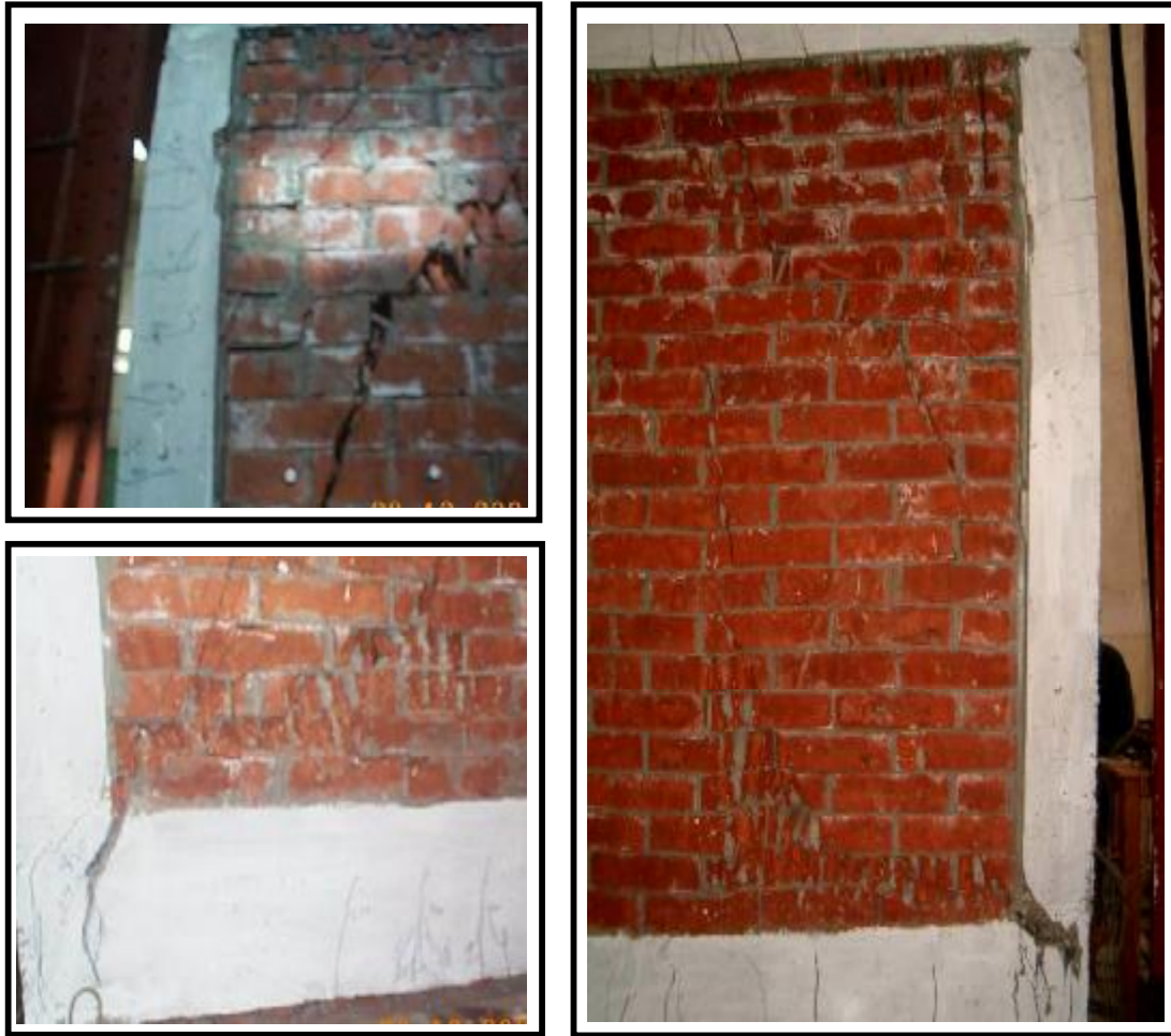
Fig. 10: Cracks Pattern and Mode of Failure for Specimen GI-2.
